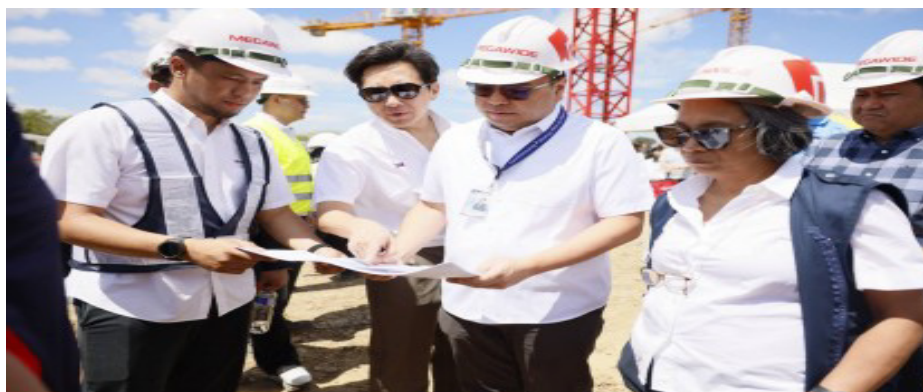
4PH PROJECT INSPECTION. Department of Human Settlements and Urban Development Secretary Jose Ramon Aliling (center) reviews site plans with Pag-IBIG Fund Chief Executive Officer Marilene Acosta (right) during the ceremonial first concrete pouring for two housing projects under the Expanded Pambansang Pabahay para sa Pilipino (4PH) Program in Dasmariñas, Cavite on Wednesday (Mar. 5, 2026). The projects are expected to generate over 7,000 housing units for working-class families. (Photo courtesy of DHSUD)
